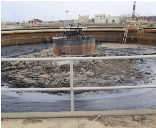
An inoperable settling tank clogged with hardened sediment found at the Back River treatment plant last March. (MDE)
